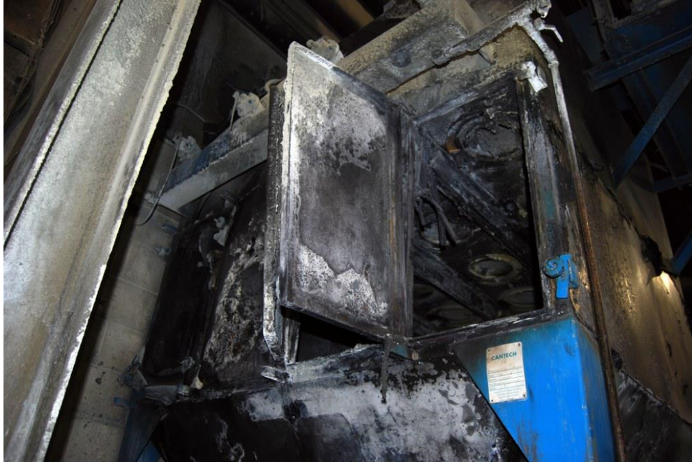
Figure 3. Fire Damaged Collector Filter Compartment
