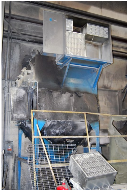
Figure 4. Dust collector after fire.
