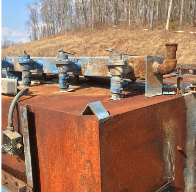
Figure 5. Compressed air header and valves at top of collector.
